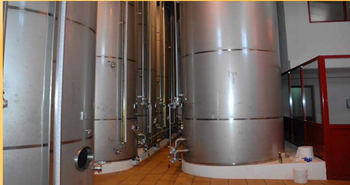
Temperature-Controlled Storage: Stainless Steel Tanks With Inert Gas (Nitrogen or Argon) system, At Montilla PLant
